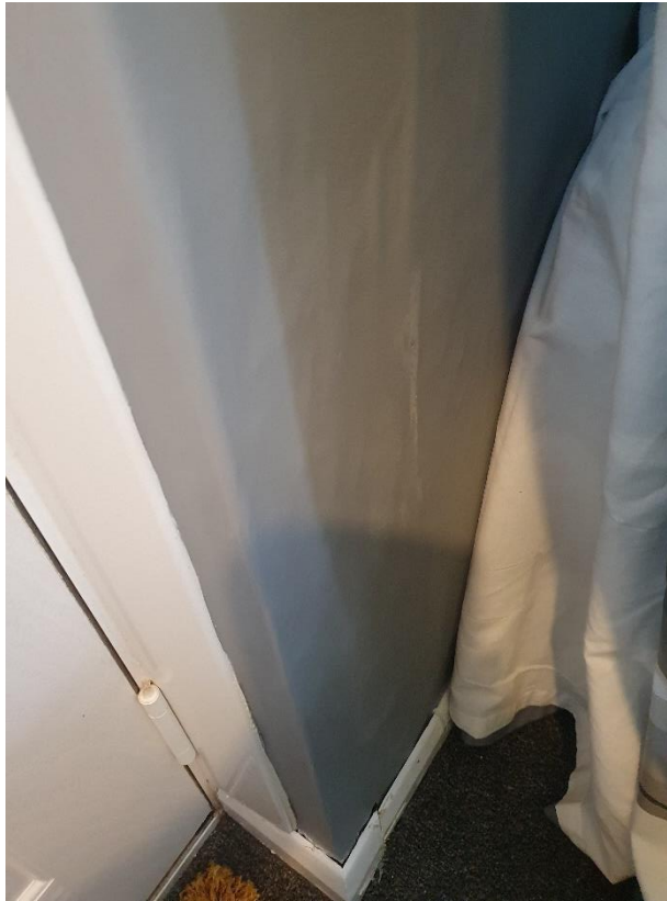
Damp to wall right of front door in lounge
