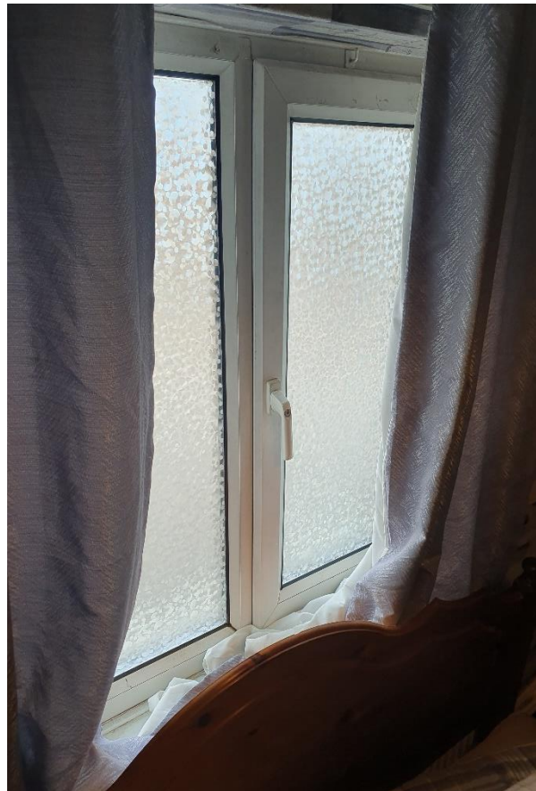
Opening inwards windows with no trickle vents
