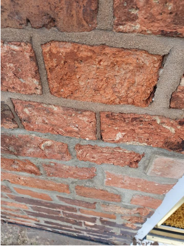
Spalling brickwork to front elevation
